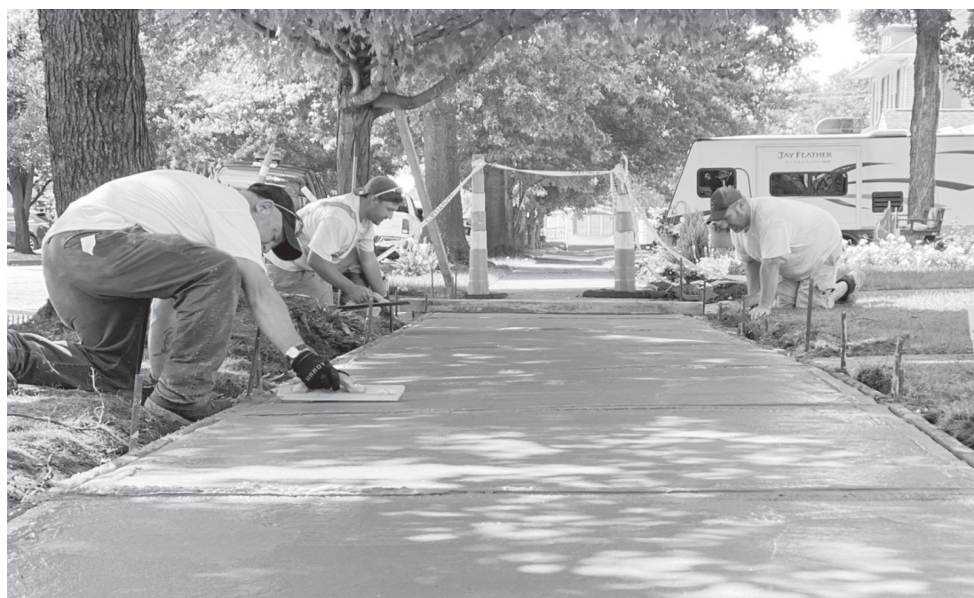
Dale Maynard, Tyler Lyons and Tim Haynie finishing a sidewalk project on B Street
