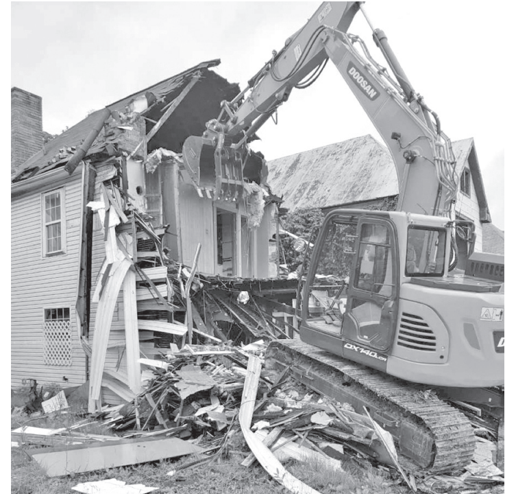
The Main Street properties have been purchased by the Golden Girls Group Home, and construction
